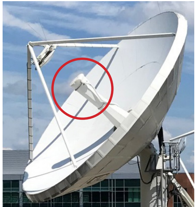
Walton De-Ice Feed Horn and Sub-reflector De-Icing System
