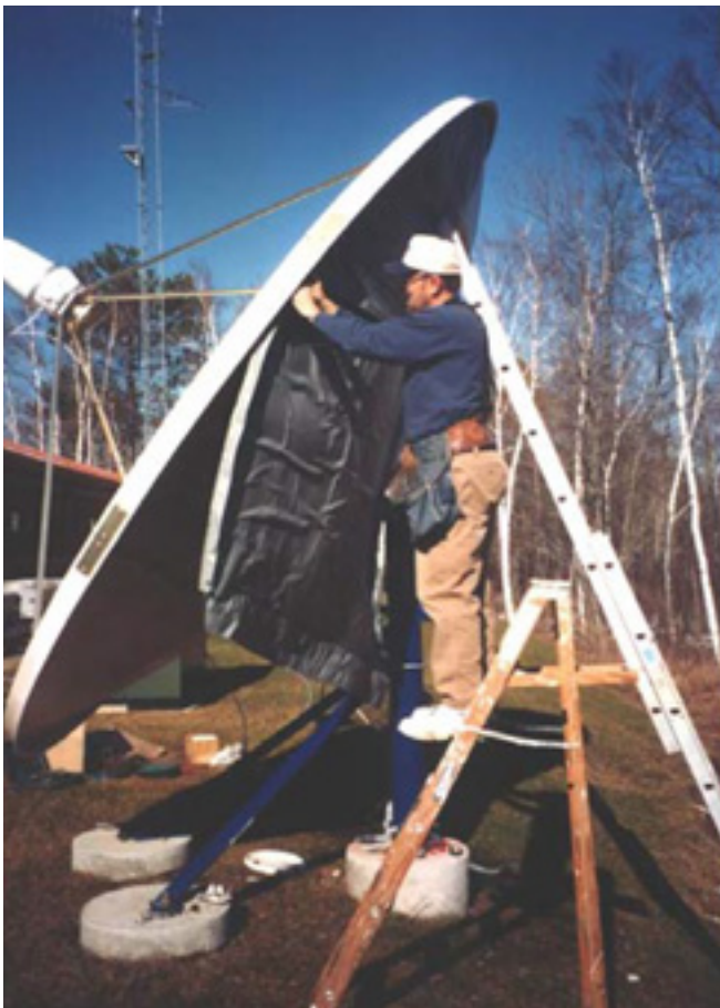
Walton Field Technician removing competitor's anti-icing system prior to installing a Walton Hot- Air De-Icing System
