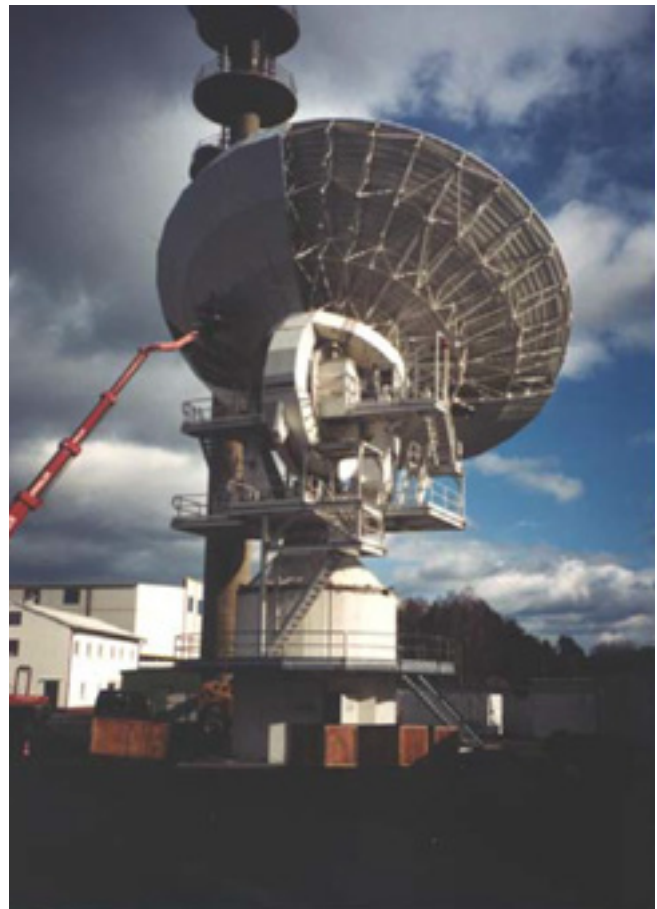
Walton Field Technicians installing a Walton Hot-Air De-Icing System on a 18 meter Antenna
