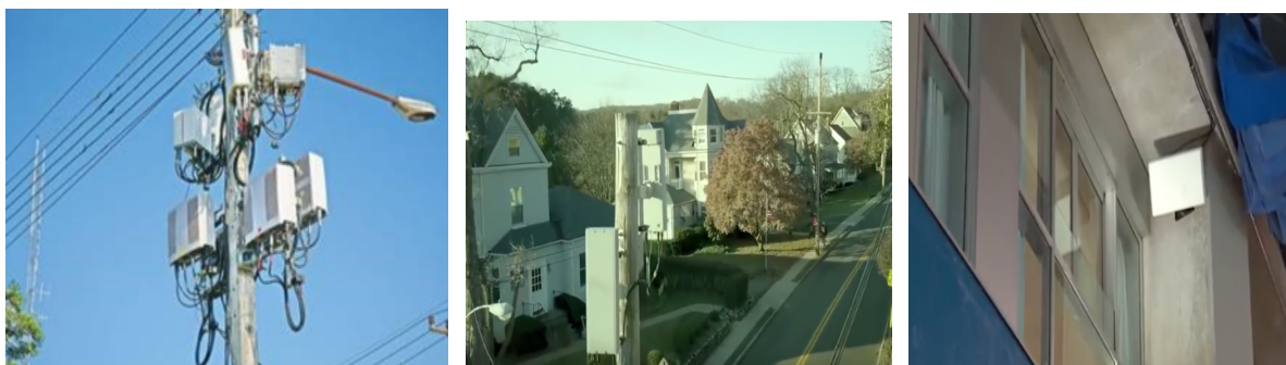
Figure 2: Small cell base stations attached to lampposts and buildings in North America
