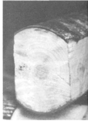
PLATE 63 The two sides hewed, the log is now ready for notching. The remainder of the sides will be hewed after the logs are all in place in the cabin.
