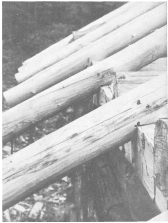
PLATE 108 The pole rafters of Thompson's log cabin are notched to fit over the plate and beside each joist.
