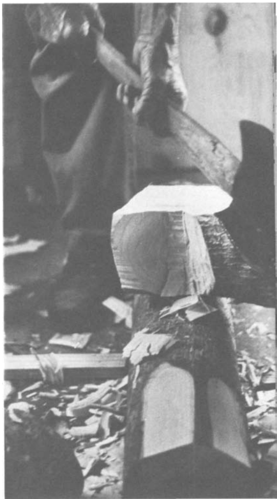
PLATE 82 Hew off two sides of the next log, rest it atop the peak of the first, and using the steel ruler as in the dovetail notches, trace the slopes of the bottom log's peak on the sides of the top log. Then hew out the notch using these lines as a guide.
