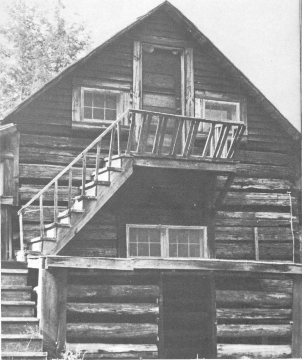
PLATE 123 The gable can be designed to hold a door and windows, as seen on this cabin at the Jay Hambidge Art Foundation in Rabun County.
