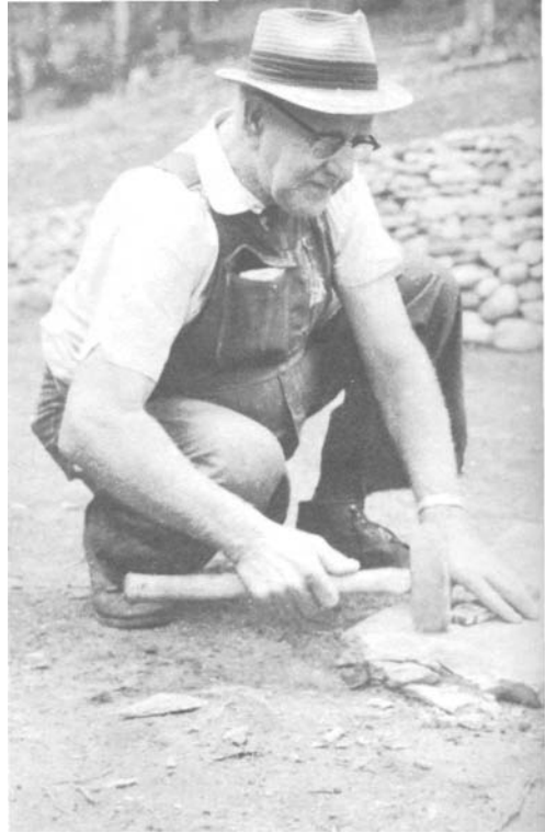
PLATE 149 Often the flagstones must be reshaped to fit. Claude measures the hole to be filled and then breaks the excess away with a hammer.
