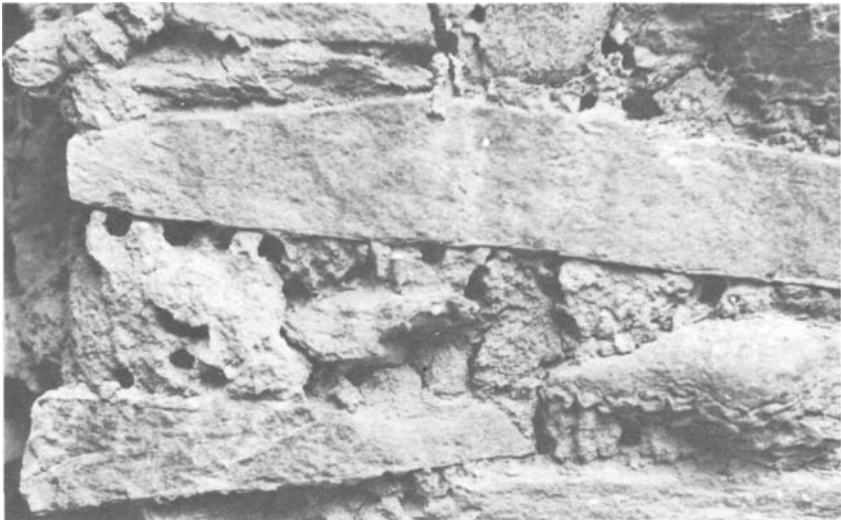
PLATE 144 A common problem with all-mud chinking was that it soon became the home for bees as the holes in this chinking show.
