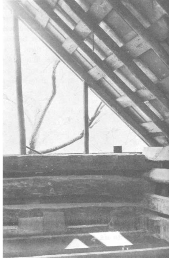
PLATE 106 The ends of these rafters are sloped and set directly on the last wall log. Note also the lathing for the roof.
