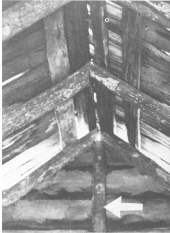
PLATE 121 From inside, center vertical support beam (arrow) for gable is visible. Note absence of ridgepole, and spacing of lathing for shingles.
