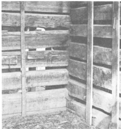
PLATE 89 The ends of this inside wall (running from left to center) have been notched to fit similar notches cut in the outside wall (running from center right).
