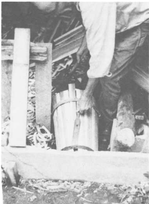
PLATE 348 A chisel can be used as shown to help fit the last stave.
