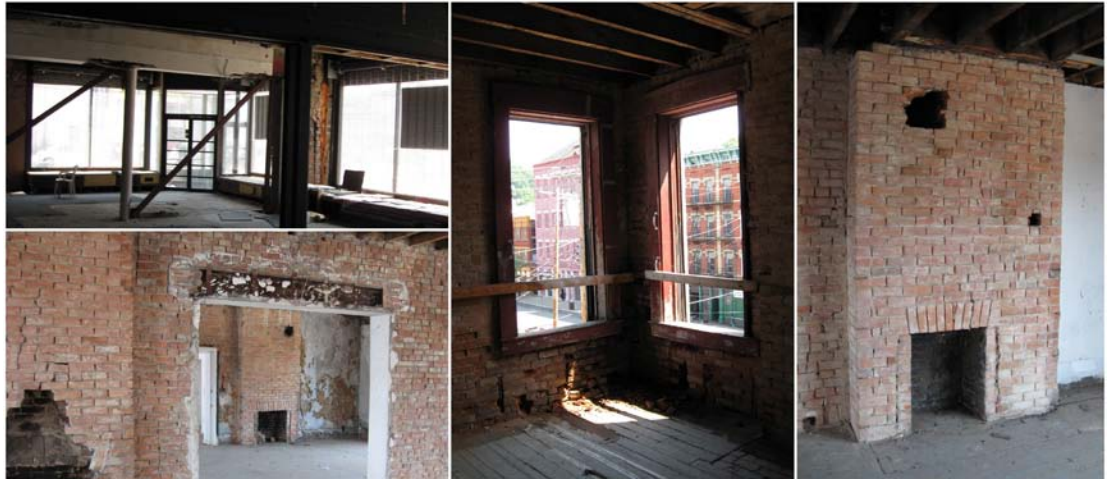
Figure 59 - 100 West Elder 'Derelict' Imagery
