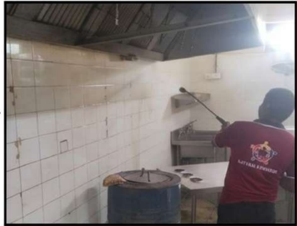
WALL & HOOD DEGREASING (KITCHEN)
