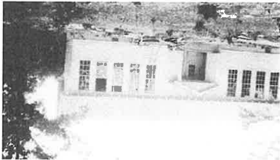
Destroyed by Fire
