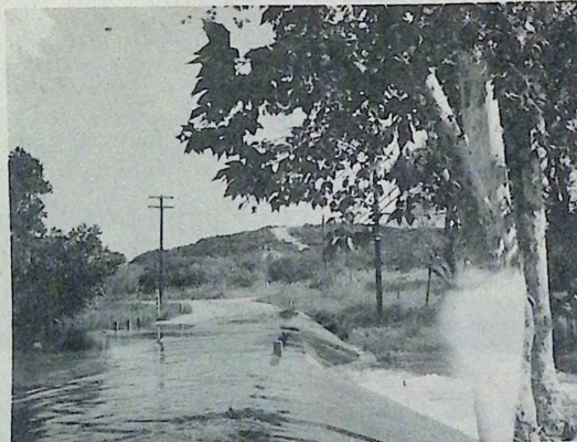
Here the Scenic Loop road Highway 16 becomes a dangerous ledge near
