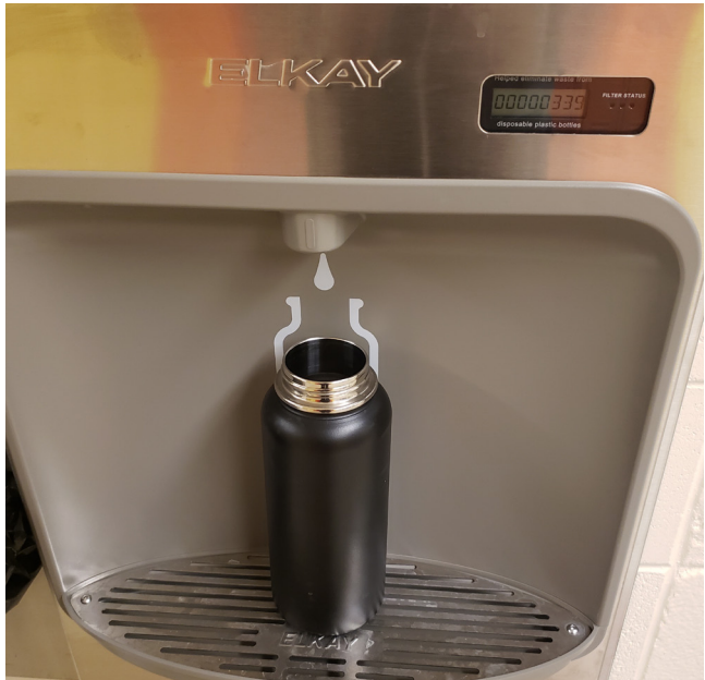
One of the new water bottle filling stations recently installed at HHS.
