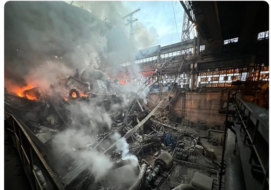
1,5 GW+ operating thermal powerplant machinery hall ruined by Russia (a state sponsor of terrorism according to the European Parliament) during missile attack on Jan 14, 2023
