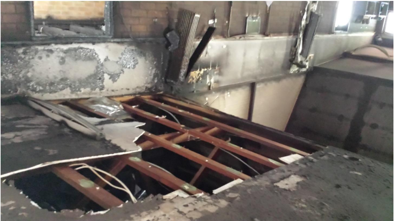
Burned roof damaging the roof
