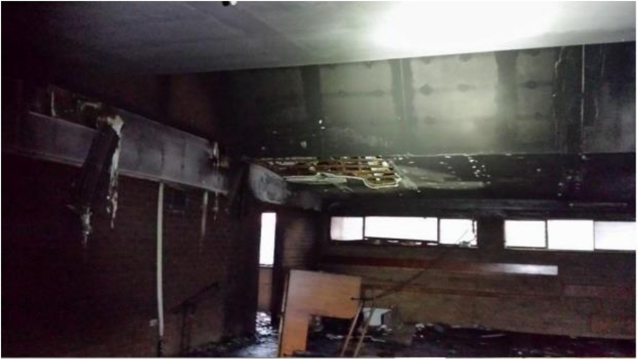
Burned ceiling and aircon machines
