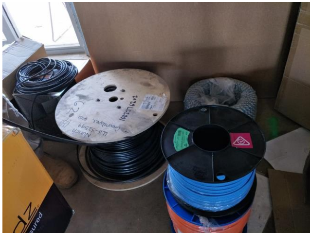
Cabling for sound system and security camera, surveillance and alarm.
