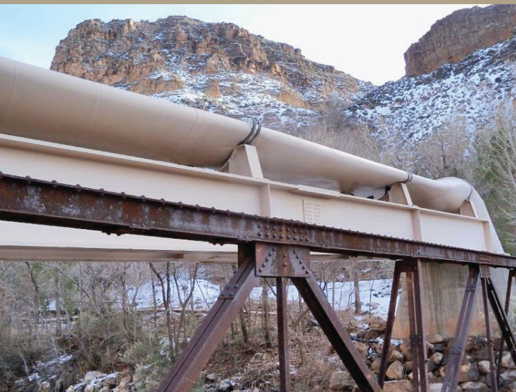
Vacuum pressure created inside pipelines while draining, in addition to air valves failures, can cause even steel pipelines to flatten like a pancake.
