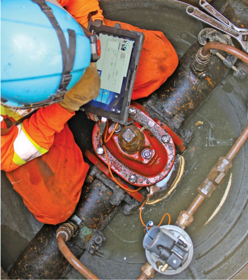
Hamilton Water staff connect to the anti-stagnation valve to set the flow schedule.
