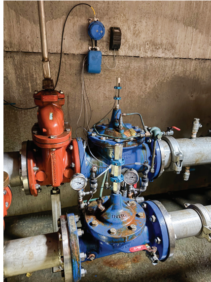
The 200 mm PRV for high-demand and the 100 mm PRV for low-flow with the Cla-Val XP2F monitoring system mounted on the wall.
