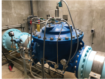
As temperatures drop, water system operators face freezing conditions that can impair or disable piloted control valves.
