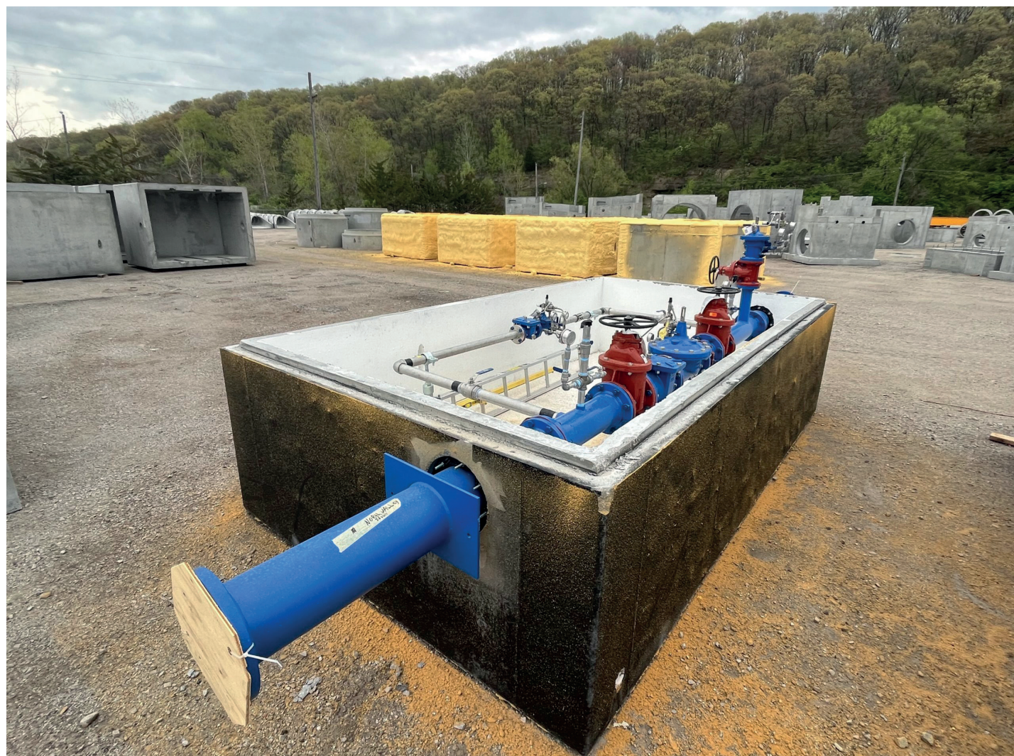
A well planned out valve station, has good access for maintenance
