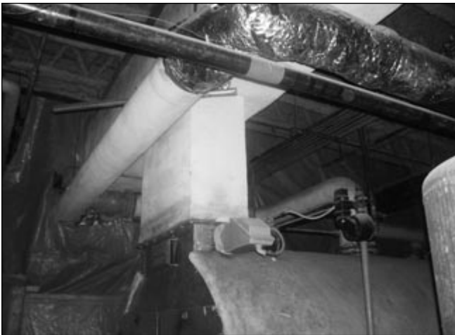
Pipe and boiler insulation
