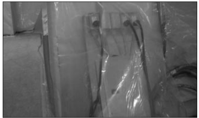
Isolated electrical panel
