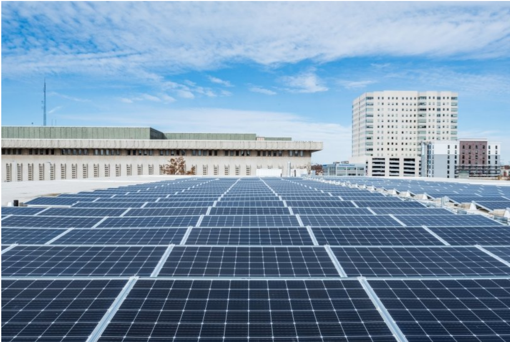
Solar PV panels atop the Tulsa Central Library provide energy in downtown Tulsa, Oklahoma. Photo courtesy of Jared Heidemann.
