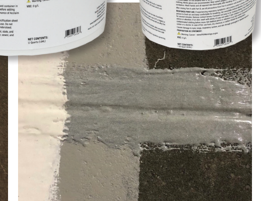
Acclaim® FSG applied by chip brush over seam on a concrete roof system prior to coatings application.
