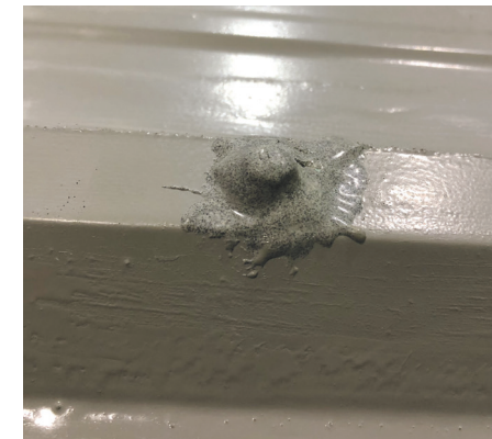
Acclaim® FSG applied by chip brush over fastener head on an R-panel metal roof system prior to coatings application.
