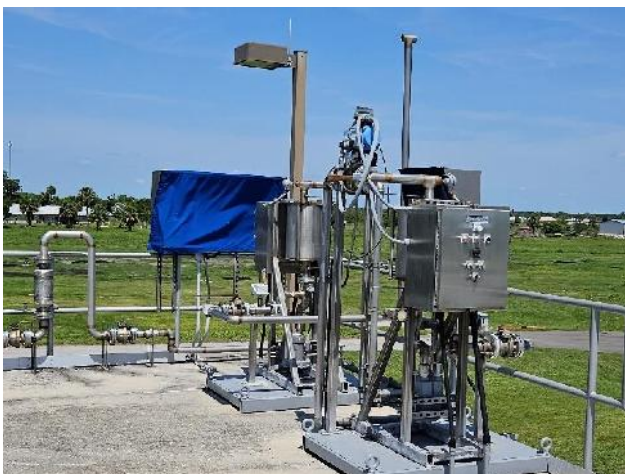
Ozone destruct Units
