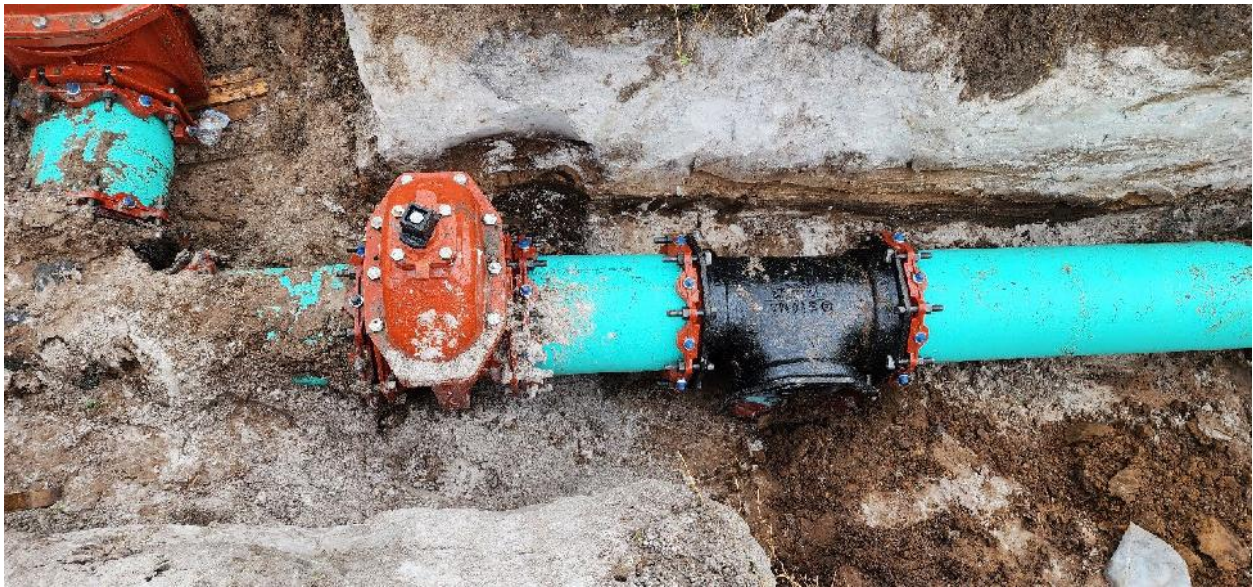
3 – 12" Gate Valves and Bypass Tee (NW-15)
