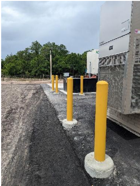
2 – Bollards Painted, Asphalt
