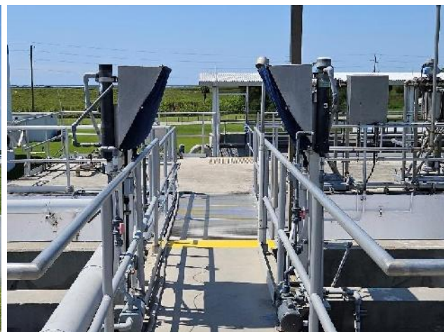
Turbidity Meter Cabinets
