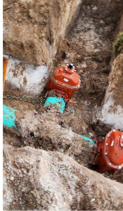
2 – 12" Gate Valves at NW-15
