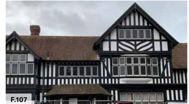
Figure 107: The Firs located on Little London built by high quality timber frame and render
