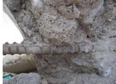
Figure 7. Detail of Pull-out failure.
