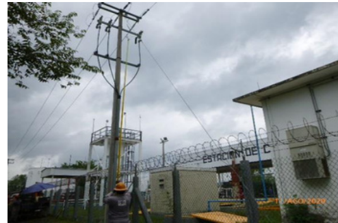
Circuit opening 13.2 kV in battery of pumping
