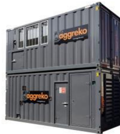
Double generation module of 1375 KW each
