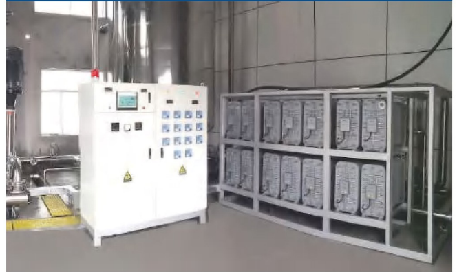
A Photovoltaic Project 70 T/H Ultrapure Water System
