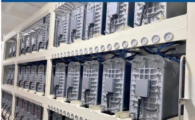
A Thermal Power Project 200 T/H Demineralized Water System
