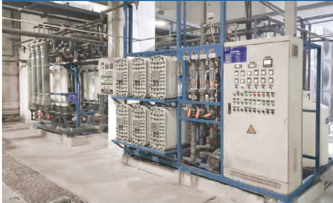
A Waste Incineration Power Generation Project 30 T/H Demineralized Water System
