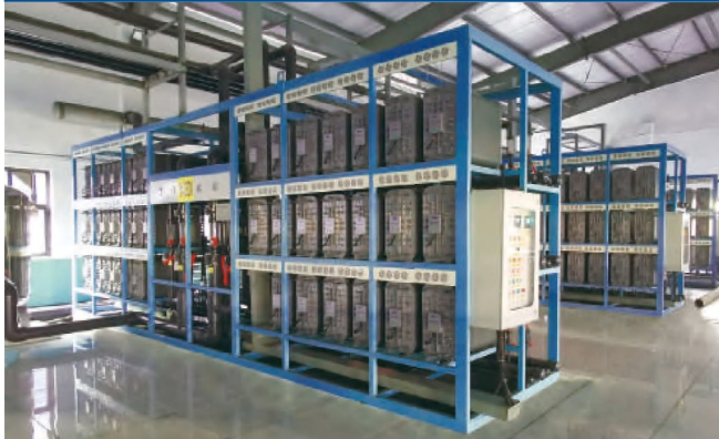
A Coking Project 3X200T/H EDI Ultrapure Water System
