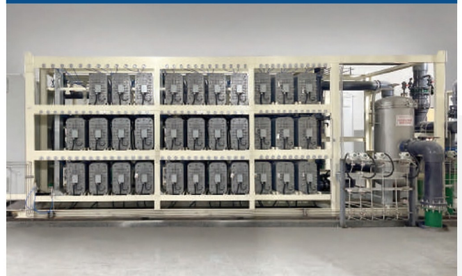
A Chemical Project 1200 T/H Demineralized Water System
