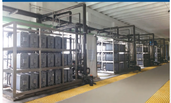
A Combined Heat and Power Project 4x100 T/H Demineralized Water System
