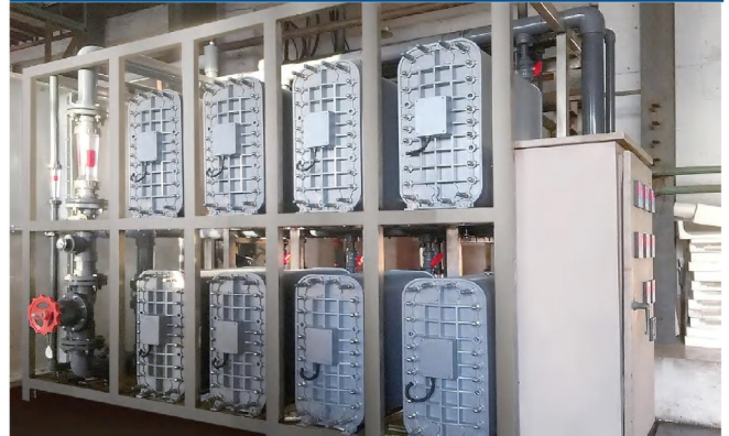
A Biomass Power Company 80 T/H Demineralized Water System
