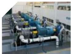
Seawater desalination project, UAE
