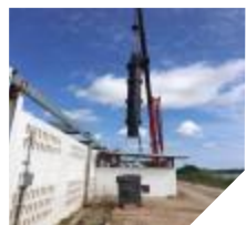
Texas flood control, USA
