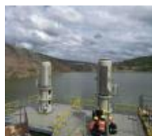
power plant, Thailand
