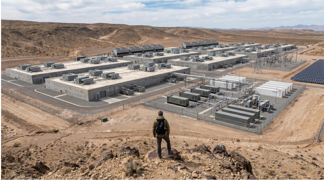
The triangle solved on one parcel: server halls beside their own substation and transmission towers (grid), on-site gas generators and fuel piping plus battery containers (firm power and fuel logistics), a solar array, and empty desert for buffer. This is what “powered land” actually looks like.
