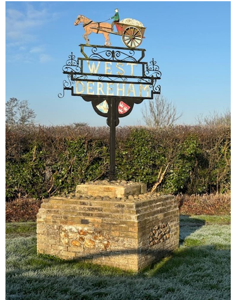
Mortar has cracked and needs renewing.
