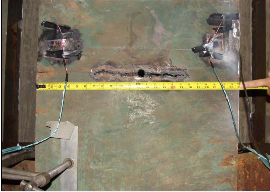
Figure 5.20: Initial cut in West RRFC main girder before fracture (looking up at bottom flange)
