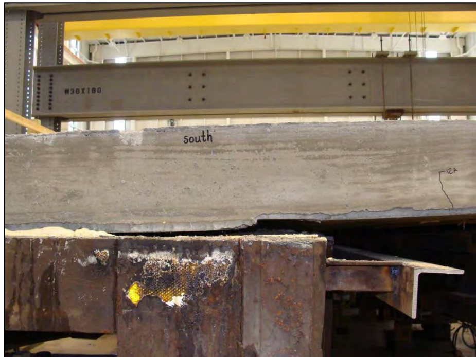
Figure 6.29: Separation of concrete deck on West RRFC
