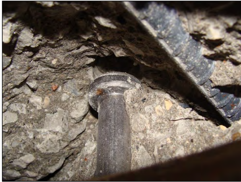
Figure 6.28: Separation of shear stud in concrete deck after Fracture Test 1
