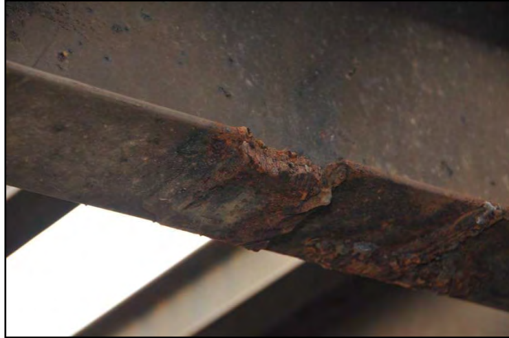
Figure 3.3: Local burn-through on bottom flange of a transverse member
