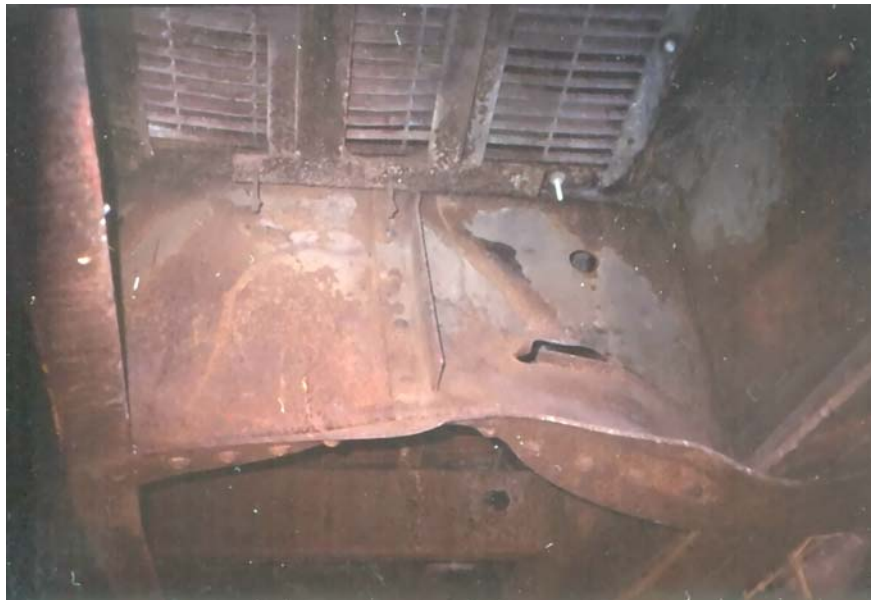
Figure 3.7. Damaged transverse member in west flatcar.
