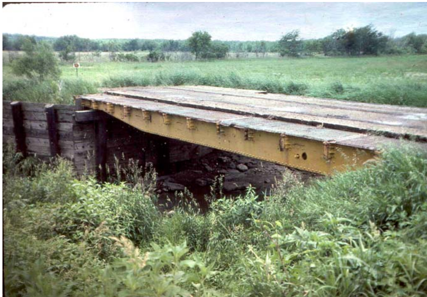
Figure 3.2. Elevation view of TCB and south abutment (Note that the girder extends past the abutment cap beam).
