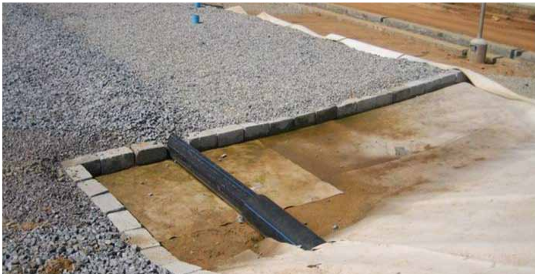
Figure 4.15: Test Field with all Sealing Components 19
