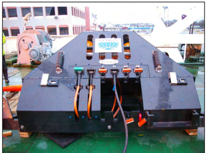
Figure 3. VENUS node installed on node base showing power input, signal input and four science ports.
