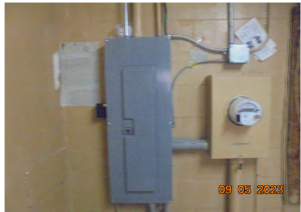
22 Mechanical Room Electrical Panel
