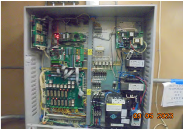
15 Elevator Control Board
