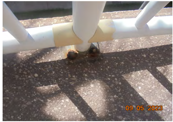
42 Above Rust Stains
