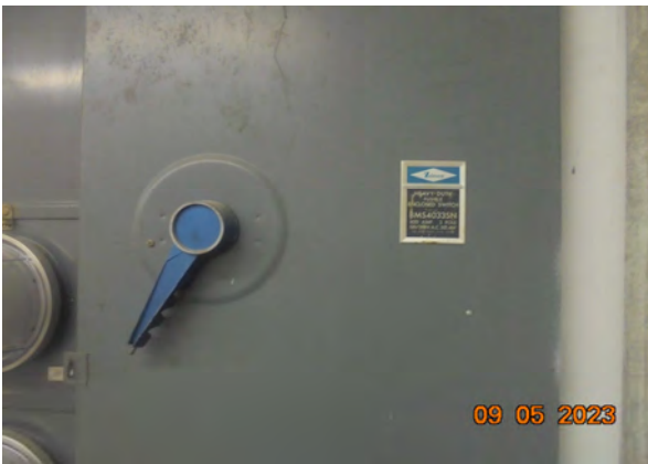
21 Main Shut Off
