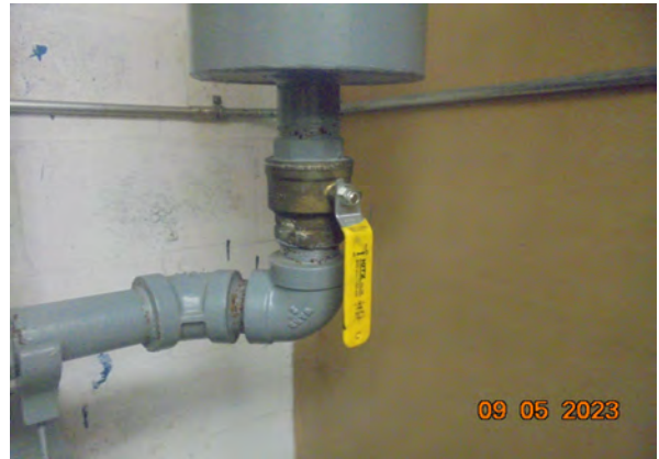
14 Elevator Pump Shut Off
