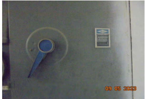
20 Main Shut Off
