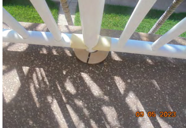
44 Above Rust Stains
