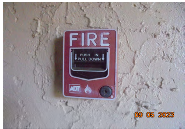
26 Fire Alarm Pull Block
