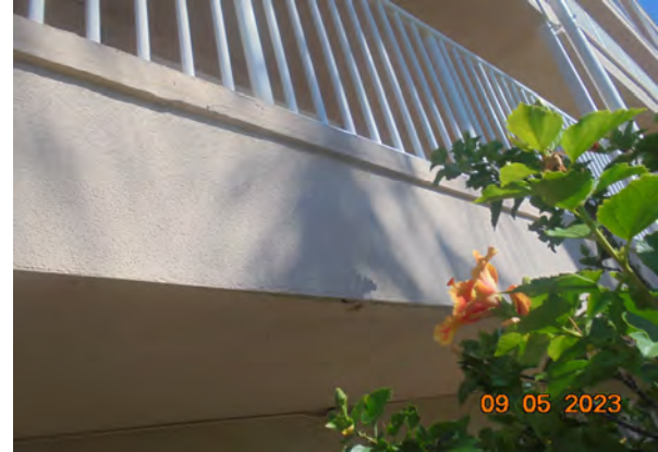
36 Delaminated Stucco Area Overview
