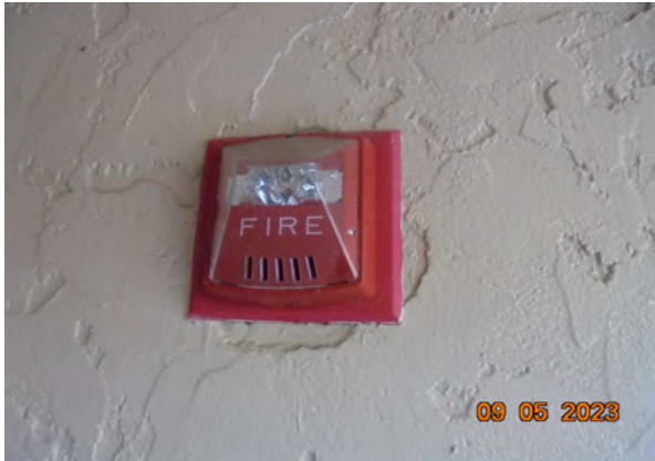
27 Fire Alarm Strobe and Siren
