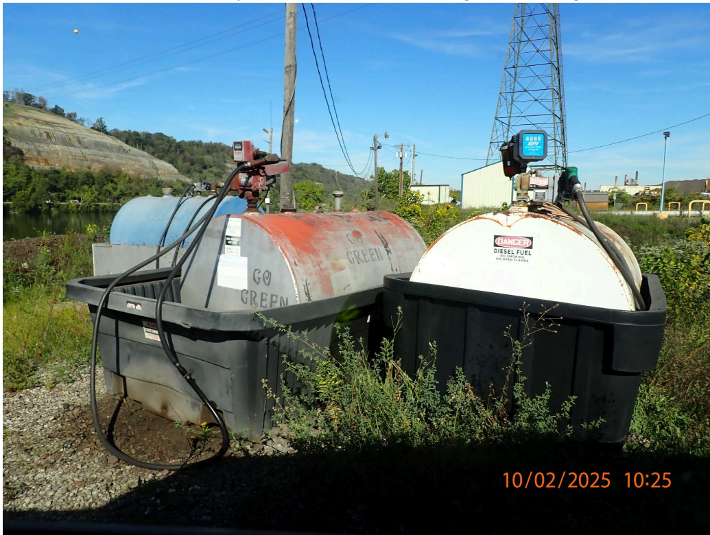
PA020332 - Middle diesel tank without a plug for secondary containment; note staining
