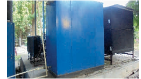
Water chilling facility
