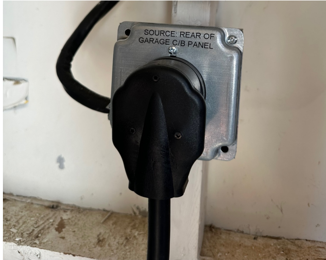
Figure 8. Home vehicle charging plug labeled for responders to know where to disable power.
