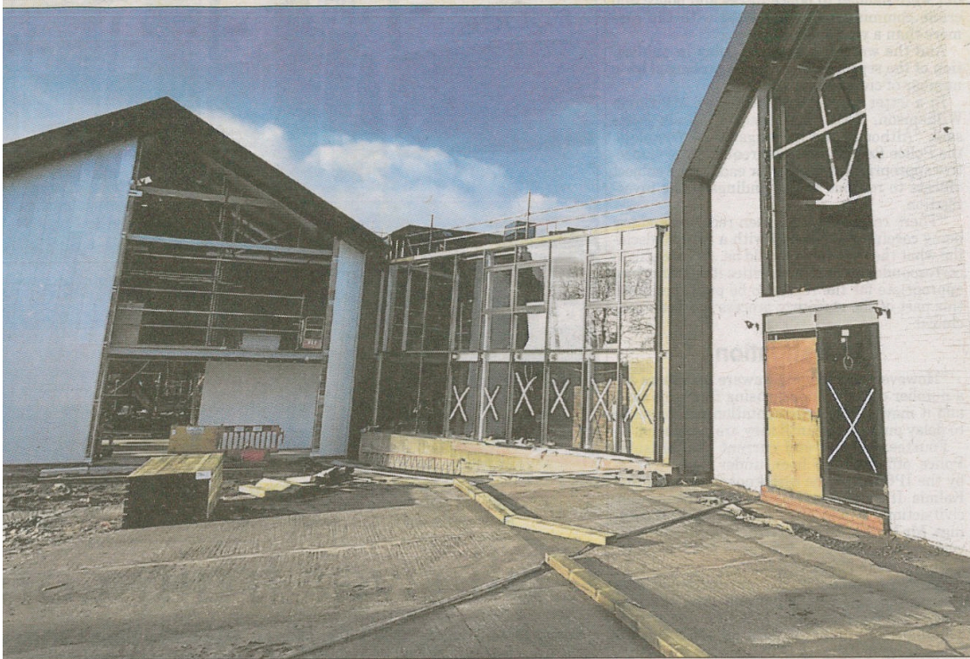
Work continues on the new Museum of Glass, Camp Hill, Wordsley, which is opposite the Red House Glass Cone attraction
