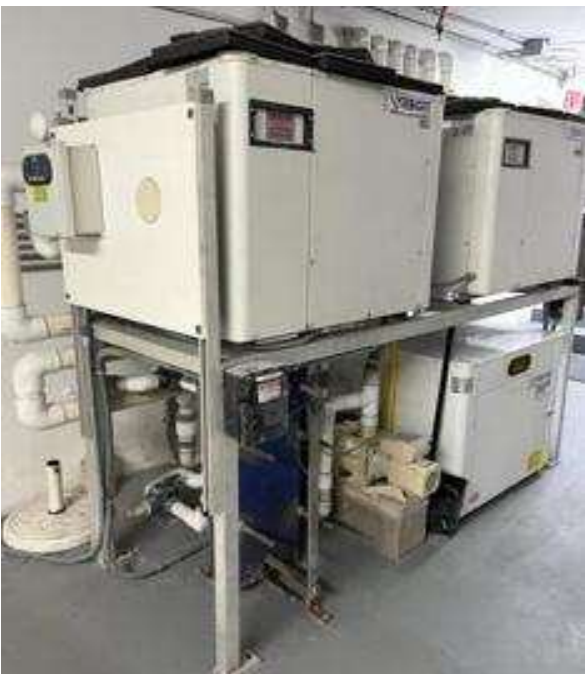
Picture #27 Pool equipment and electrical connections are good.
