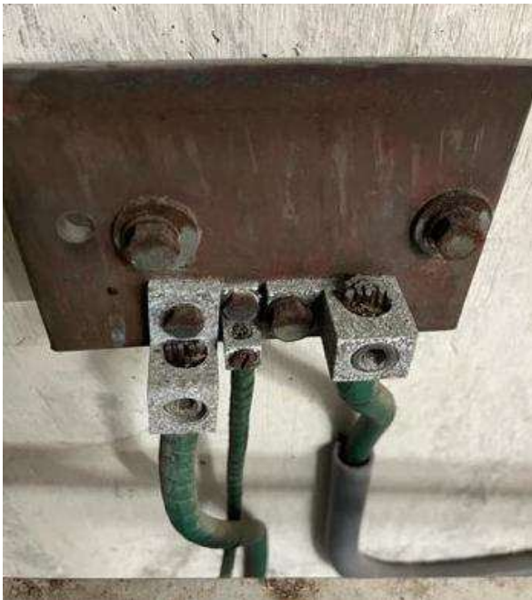
Picture #25 Grounding system is good.
