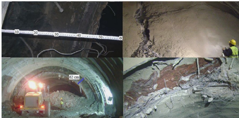
Fig. 7. The view of the deformed T13 tunnel.
