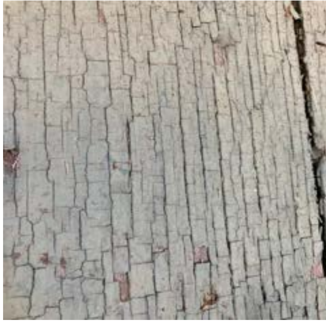
Figure 4 – Detail of barn door paint.
