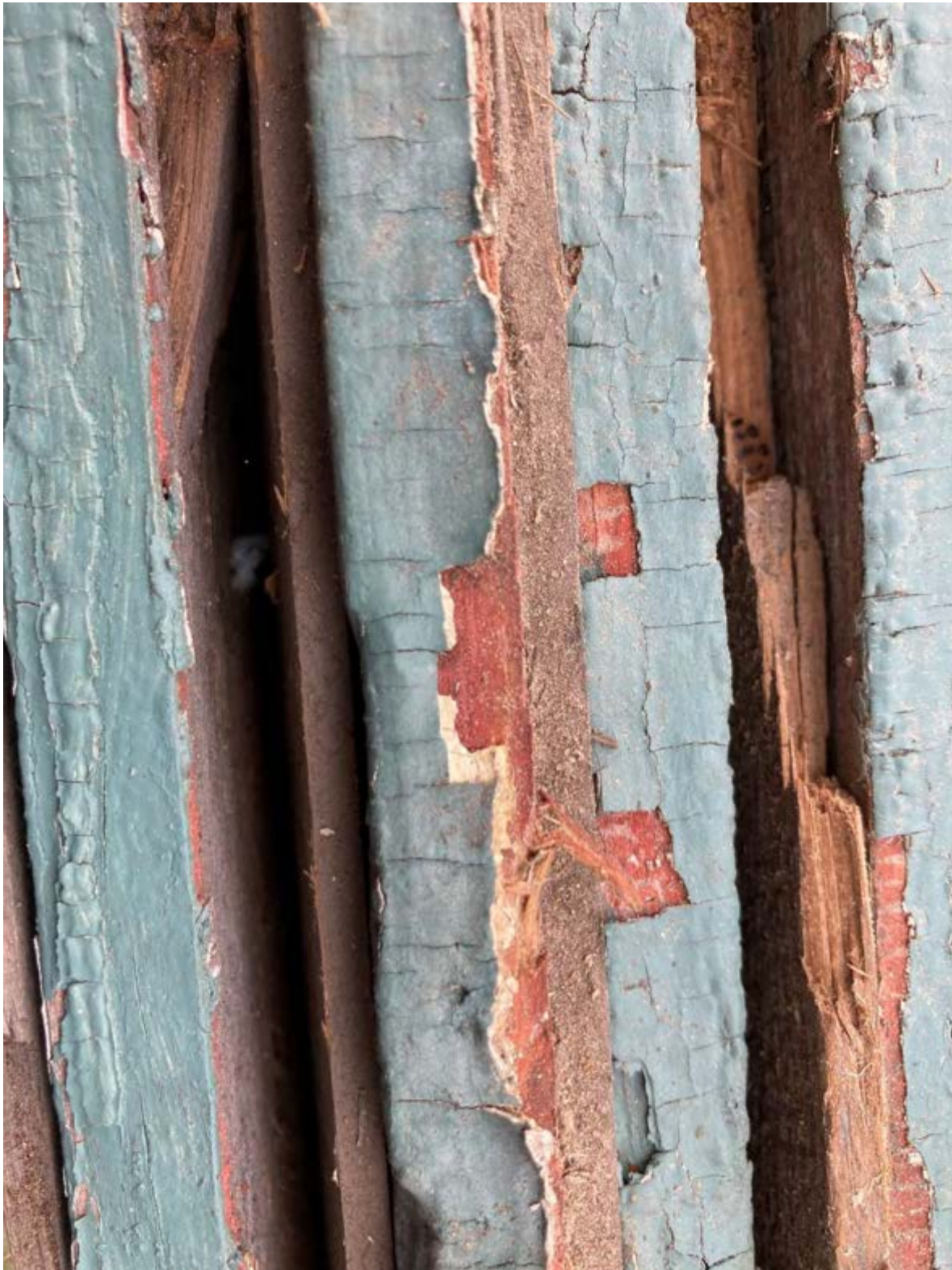
Figure 11 – Detail of siding showing color layers.
