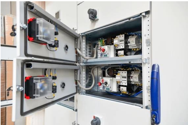
Figure 1: Protection & Control Relays
