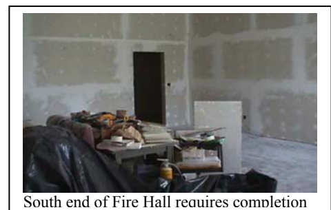
South end of Fire Hall requires completion
