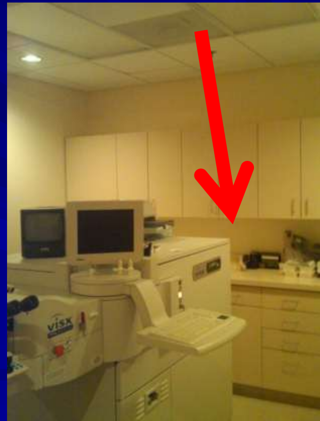
Air duct in laser room
