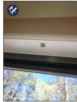
Minor Damage Observed to Window Framing
