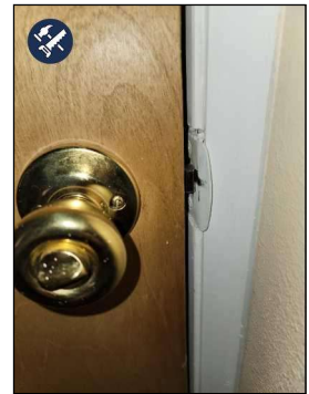
Master Bedroom#1--Bedroom Door does not Latch
