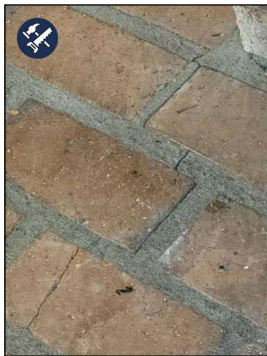
Living Room--Cracked or Deteriorated Mortar Observed in Hearth
