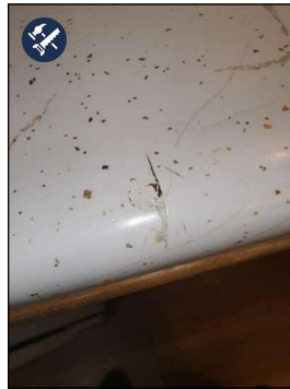
The counter tops are noted as being chipped.
