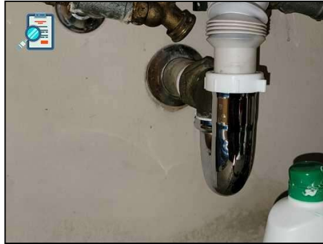
Bathroom#2--Older style metal traps noted. Buyer is cautioned that these traps can leak at any time due to corrosion.
