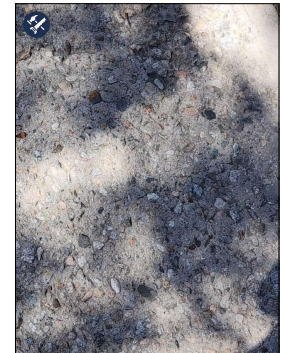
Concrete spalling noted at driveway. This loosening of the top, smooth layer of the cement is a common occurrence, possibly due to an improper curing process, age, or use of snow-melting materials.
