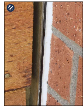
Sealant Between Chimney and the Home is Cracked/Broken or Missing.
