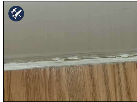
Master Bathroom#1--Recommend caulking at the tub and shower areas
