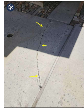
Moderate cracks in driveway. Repair and / or monitor for expansion and development of trip hazards.
