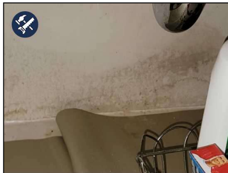
Bathroom#2--There appears to be water damage under sink. This tested dry at the time of the inspection, but monitor for any further intrusion.
