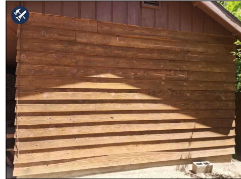
Peeling Finish observed, suggest scraping and Re-Staining as necessary. Most of the South Side.
