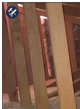
Daylight Visible by Chimney Bricks
