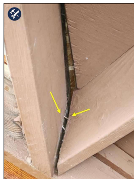
South Side Rear Porch Area above Roofing Components are Separating. Above Water Heater Closet.
