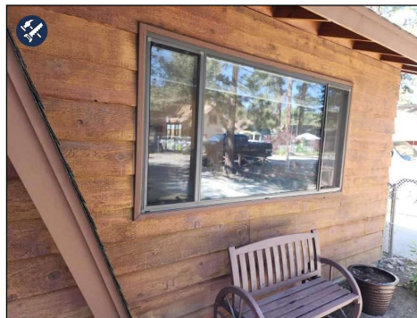
Peeling Finish observed, suggest scraping and Re-Staining as necessary. Most of North Side.
