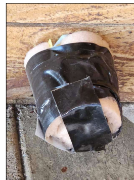
Appears Functional. South Side.
