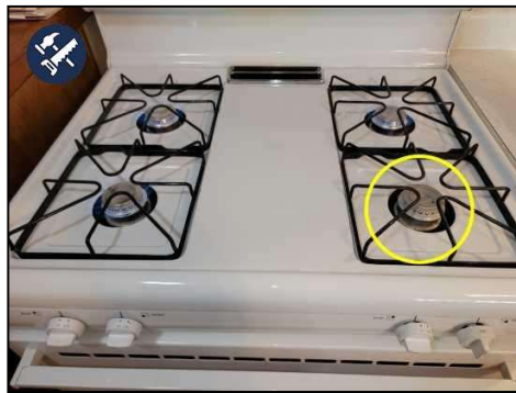
1 burner did not operate properly when tested.
