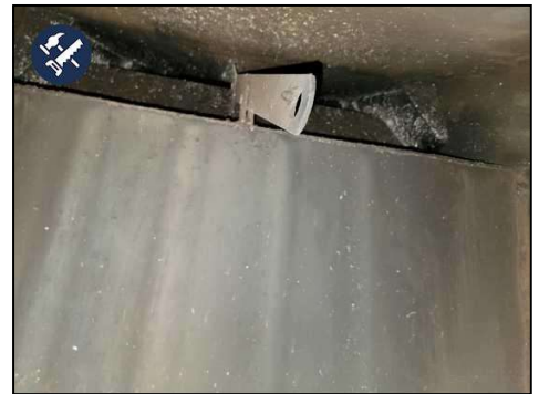
Living Room--Flue Damper is Stuck Open
