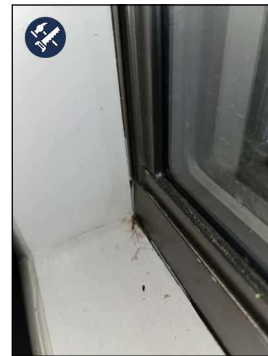
Living Room--Cracked Seal Observed around Window Framing
