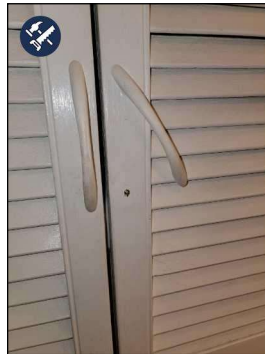
Loose Handle Observed
