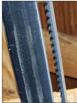
Belt drive opener noted.
