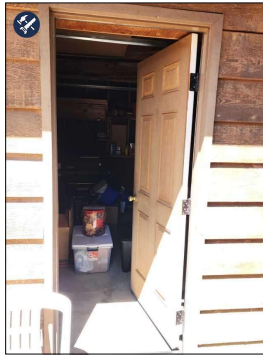
Garage Exterior Door has Peeling Finish and Bare Wood Observed.
