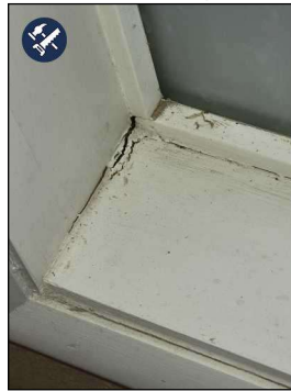
Master Bedroom#1--Deterioration noted due to contact with moisture, repairs needed.
