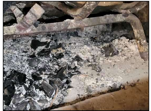
Living Room--Gas Assist Lighting Noted
