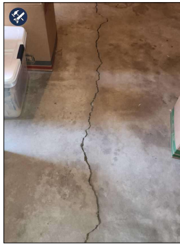
Crack entire Length Down Center Noted.
