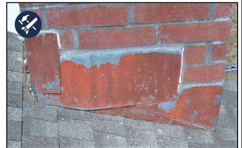
Step Flashing should be completely secured to Chimney.
