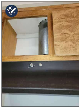
Exhaust fan is noisy.
