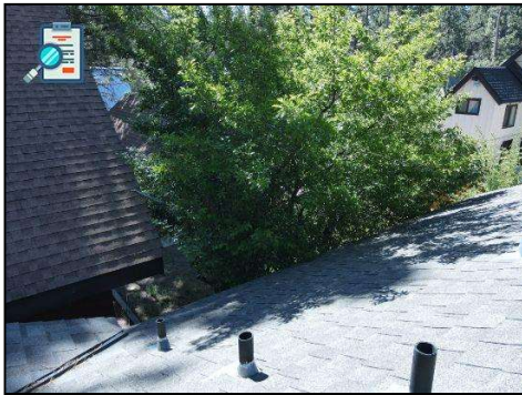
Tree branches overhanging roof and/or against siding. Trim trees that are in contact or proximity to home, as branches can abrade siding and damage roofing.
