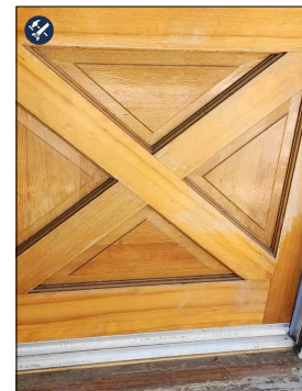
Peeling Finish observed, suggest scraping and Re-Staining as necessary. North Front Entry Door.
