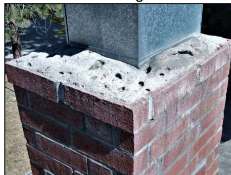
Concrete Crown is all Pitted and Cracked Up. Recommend further evaluation by a Roofing Contractor or Chimney Specialist for Answers & Options to this Issue.
