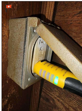
GFCI Receptacle would not Trip When Tested. Made a loud humming sound but no trip. Recommend Replacing Receptacle. South Side Right Side of the Water Heater Closet.
