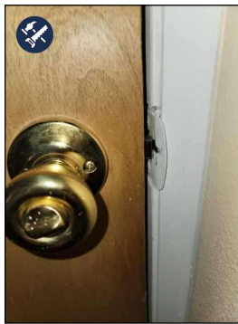
Master Bedroom#1--Bedroom Door does not Latch
