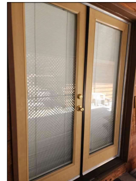
Appeared in functional and in satisfactory condition, at time of inspection. West Side.
