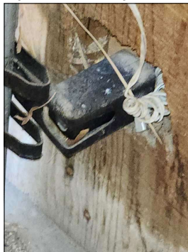
Eye beam system present and operating.
