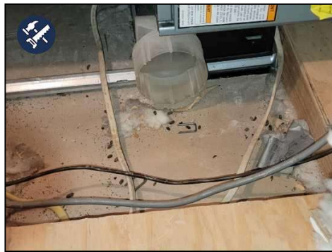
Evidence of Rodent Activity Observed
