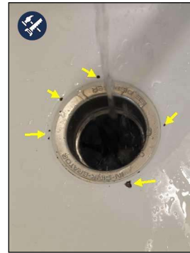
Sink chipped (Cosmetic; does not affect function).
