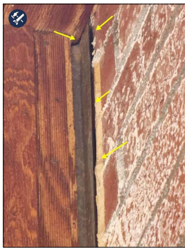
Sealant Between Chimney and the Home is Cracked/Broken or Missing.
