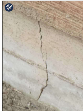
Cracks and deterioration observed. North Side.
