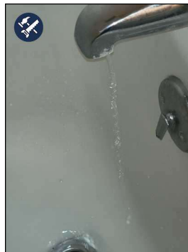
Bathroom#2--Shower diverter does not fully engage.
