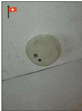
Master Bedroom#1--Replace all old not functioning smoke/ fire detectors with new hard wired detectors or make sure batteries are good.
