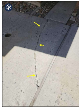
Moderate cracks in driveway. Repair and / or monitor for expansion and development of trip hazards.
