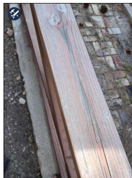
Peeling Paint and Bare Wood Observed. East Side Fencing.
