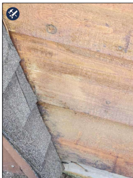
Peeling Finish observed, suggest scraping and Re-Staining as necessary. North Side.
