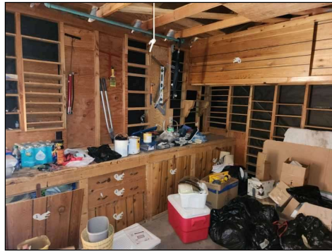
There are no firewalls present.
