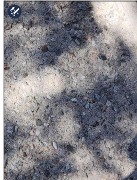
Concrete spalling noted at driveway. This loosening of the top, smooth layer of the cement is a common occurrence, possibly due to an improper curing process, age, or use of snow-melting materials.
