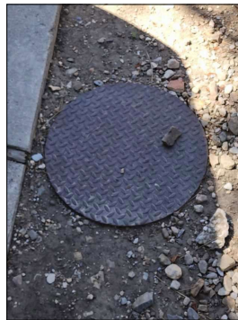
No Apparent Issues with the City Main Water Valve. Northwest Corner of the property Right of the Driveway.
