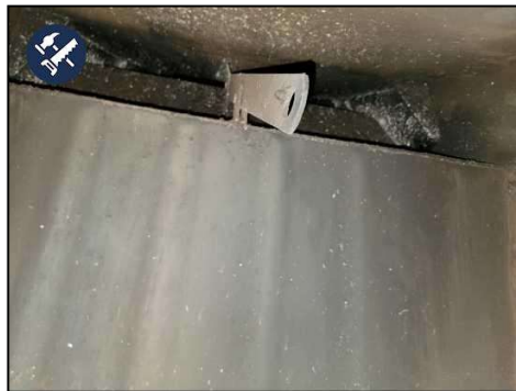
Living Room--Flue Damper is Stuck Open
