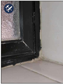
Bathroom#2--Cracked Seal Observed around Window Framing
