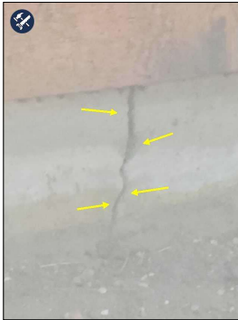
Cracks and deterioration observed. North Side.
