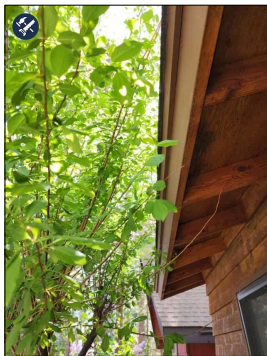
Trim trees that are in contact or proximity to home, as branches can abrade roofing or siding. North Side.
