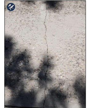
Moderate cracks in driveway. Repair and / or monitor for expansion and development of trip hazards.
