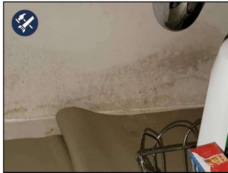
Bathroom#2--There appears to be water damage under sink. This tested dry at the time of the inspection, but monitor for any further intrusion.
