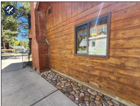
Peeling Finish observed, suggest scraping and Re-Staining as necessary. Most of the West Side.
