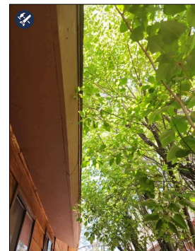
Trim trees that are in contact or proximity to home, as branches can abrade roofing or siding. East Side.
