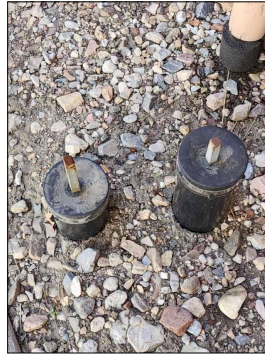
Multiple Stop & Waste Valves all working Correctly.
