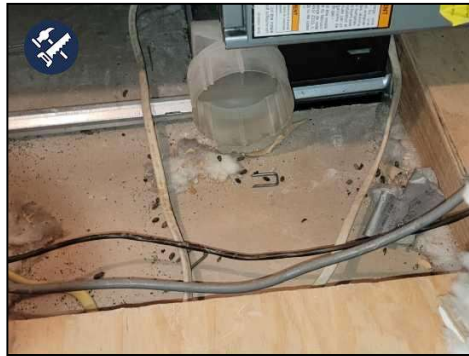
Evidence of Rodent Activity Observed
