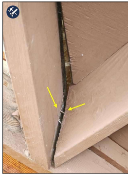
South Side Rear Porch Area above Roofing Components are Separating. Above Water Heater Closet.
