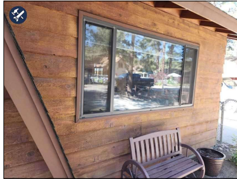
Peeling Finish observed, suggest scraping and Re-Staining as necessary. Most of North Side.
