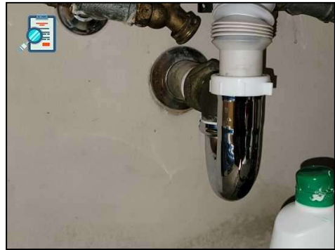
Bathroom#2--Older style metal traps noted. Buyer is cautioned that these traps can leak at any time due to corrosion.
