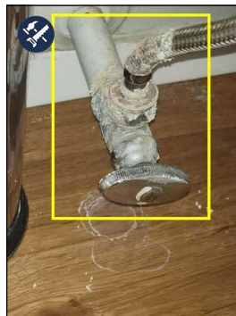
Bathroom#2--Excessive corrosion on water shutoff valve. Valve could leak at any time or may not work properly when used. Recommend further evaluation by licensed plumbing professional.
