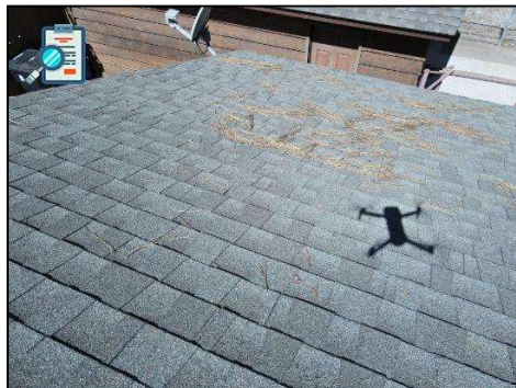
Clean Tree Debris Whenever Possible.
