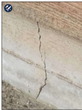
Cracks and deterioration observed. North Side.
