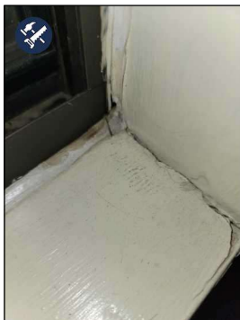
Bedroom#3--Cracked Seal Observed around Window Framing
