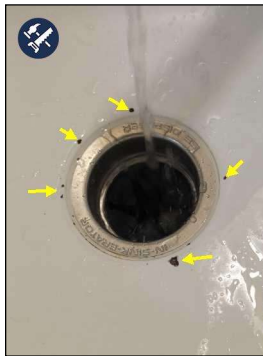
Sink chipped (Cosmetic; does not affect function).
