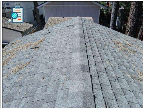
Clear Tree Debris Whenever Possible.
