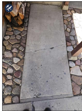
Minor Crack in The Walkway Observed. West Side From Driveway to South Side Back Door.
