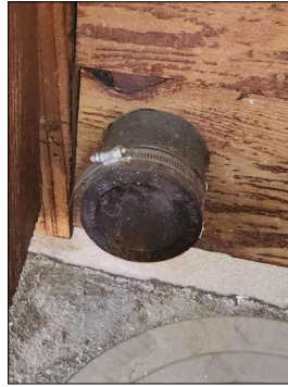
The Clean Out was Observed. South Side Right of Water Heater Closet.
