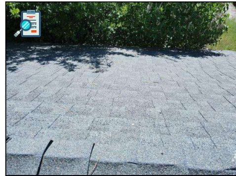
Tree branches overhanging roof and/or against siding. Trim trees that are in contact or proximity to home, as branches can abrade siding and damage roofing.
