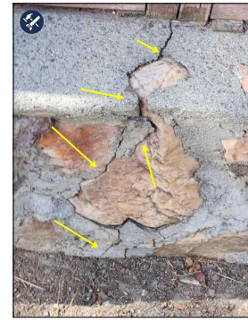
Crack in the Garden Wall Mortar. North Side.
