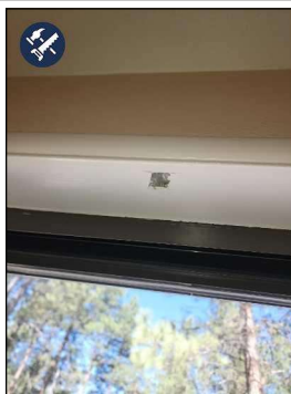
Minor Damage Observed to Window Framing
