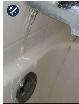
Master Bathroom#1--Tub Spout leaks while operating
