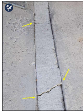
Extensive cracks in driveway. Repair and / or monitor for expansion and development of trip hazards.
