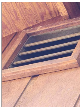
Vent screens noted as functional. East Side.
