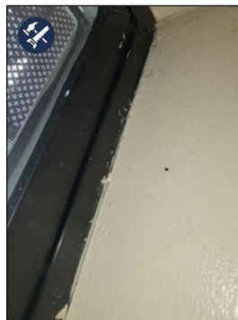
Master Bedroom#1--Cracked Seal Observed around Window Framing
