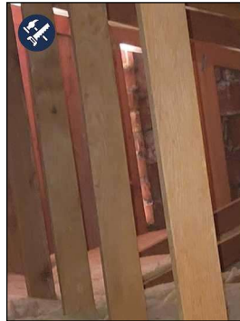
Daylight Visible by Chimney Bricks
