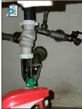
Bathroom#2--Flex drain observed, these are subject to frequent clogging.
