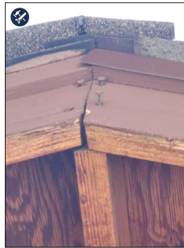
Nail Observed coming out of the Fascia Board. West Side. Another Observation, Drip Edge Flashing is only installed on the Center Sides to South Side Roofing Only!
