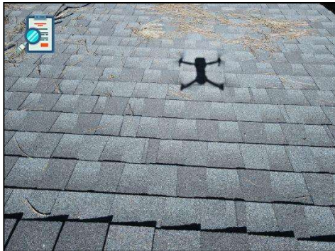
Clear Tree Debris Whenever Possible.
