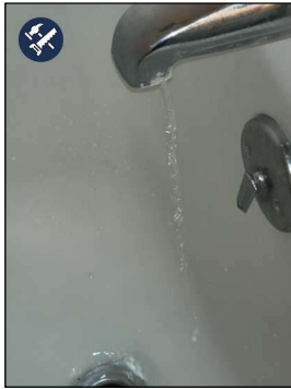
Bathroom#2--Shower diverter does not fully engage.
