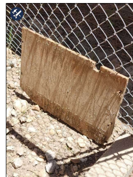
Entry Door is a Riddled piece of Plywood and should be replaced.
