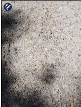
Concrete spalling noted at driveway. This loosening of the top, smooth layer of the cement is a common occurrence, possibly due to an improper curing process, age, or use of snow-melting materials.
