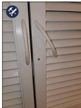
Loose Handle Observed
