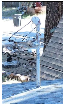
There is an overhead service drop noted.
