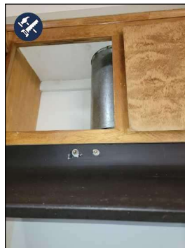
Exhaust fan is noisy.
