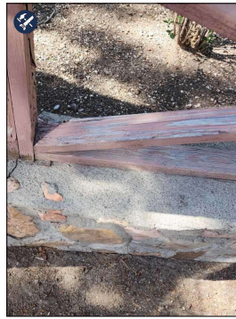
Peeling Paint and Bare Wood Observed. North Side.
