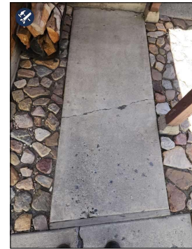
Minor Crack in The Walkway Observed. West Side From Driveway to South Side Back Door.
