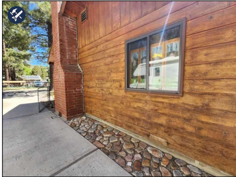
Peeling Finish observed, suggest scraping and Re-Staining as necessary. Most of the West Side.
