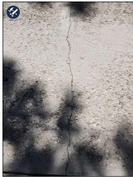
Moderate cracks in driveway. Repair and / or monitor for expansion and development of trip hazards.
