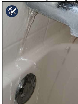
Master Bathroom#1--Tub Spout leaks while operating
