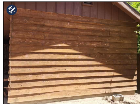
Peeling Finish observed, suggest scraping and Re-Staining as necessary. Most of the South Side.
