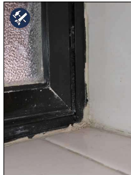
Bathroom#2--Cracked Seal Observed around Window Framing
