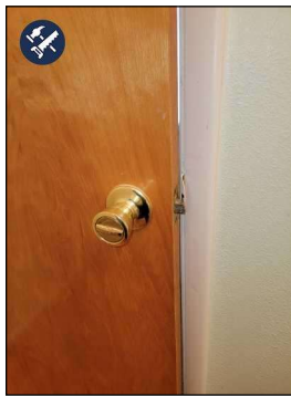
Master Bathroom#1--Door doesn't latch properly.
