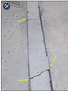
Extensive cracks in driveway. Repair and / or monitor for expansion and development of trip hazards.
