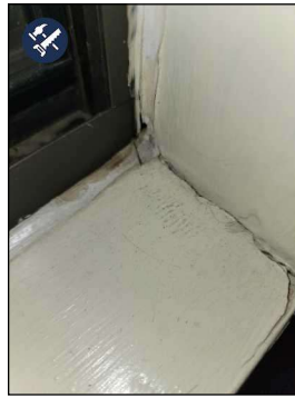
Bedroom#3--Cracked Seal Observed around Window Framing
