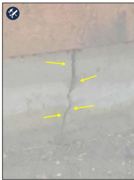
Cracks and deterioration observed. North Side.
