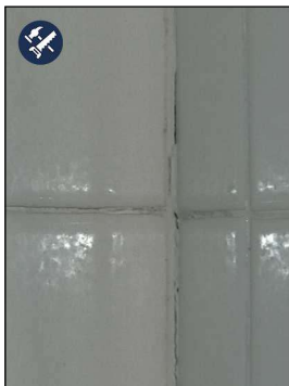
Bathroom#2--Missing/damaged grout observed, suggest regrouting as necessary.
