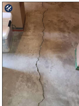
Crack entire Length Down Center Noted.
