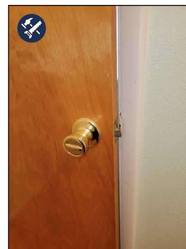
Master Bathroom#1--Door doesn't latch properly.
