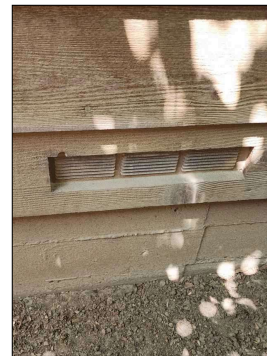
Vent screens noted as functional. East Side.
