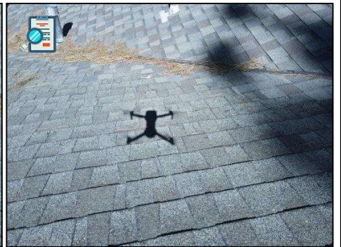
Clear Tree Debris Whenever Possible
