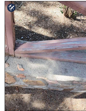
Peeling Paint and Bare Wood Observed. North Side.
