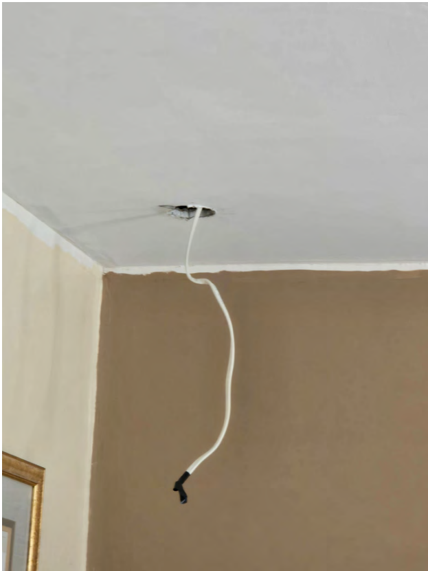
Front den has a hanging wire, and missing trim or unpainted border.
