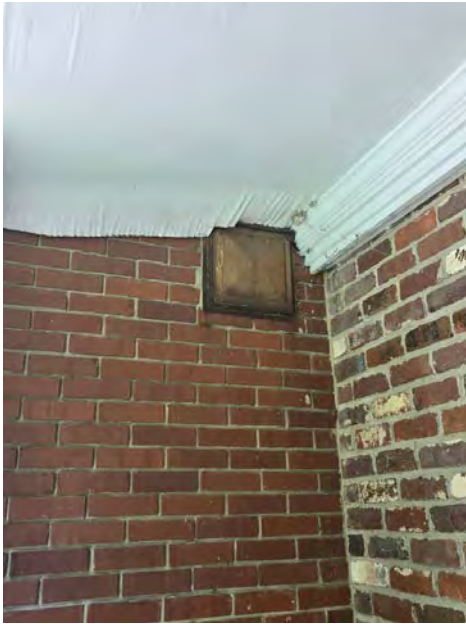
No info about this metal square. Ceiling panels are drooping on South end porch.
