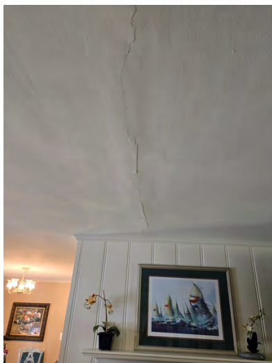
Various plaster cracks, as seen in Living Room.
