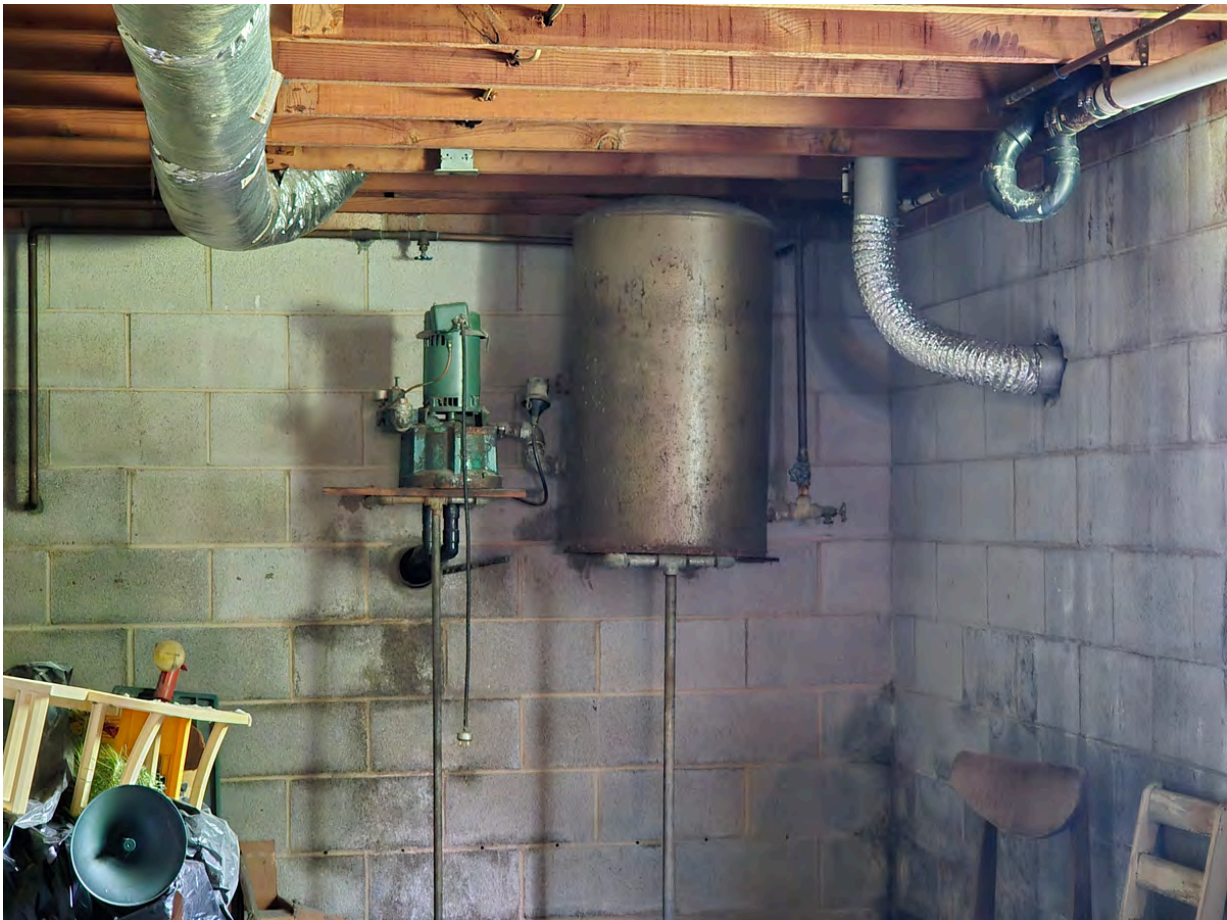
This is an old residential well water pump system. Not sure if it is in use, doubtful. I believe there may be an abandoned well somewhere on the property, but I didn't find it. House now serviced by Davidson Water.
