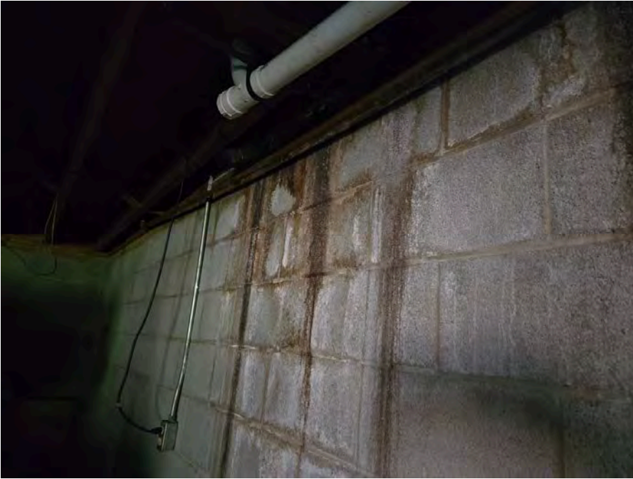
Uncertain of what this is on basement wall opposite carport in basement.
