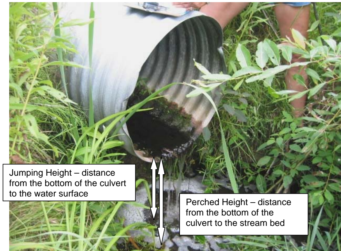
Figure 6. Measuring depth to bed of perched culvert and jumping height for fish.
