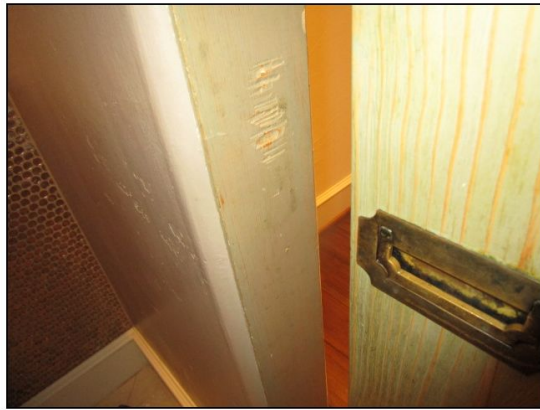
The front door does not seal on the bottom when shut.
