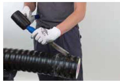
(3) Split the casing pipe with a knife or chisel. Note: Ensure you don't damage the service pipe.
