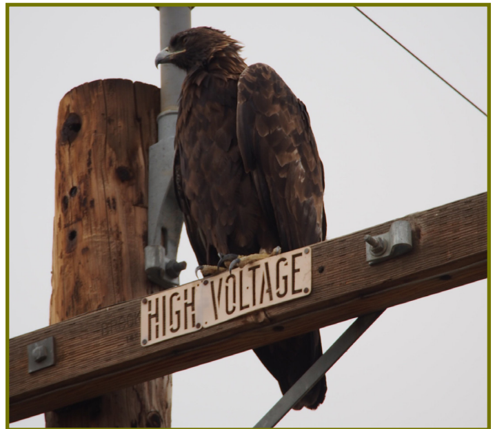
Power lines cause electrocution and collision deaths of Golden Eagles, both of which have been documented most extensively in western populations. J. Maughn, Creative Commons
